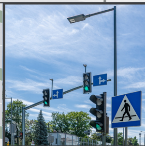
PEDESTRIAN CROSSING LIGHTING
